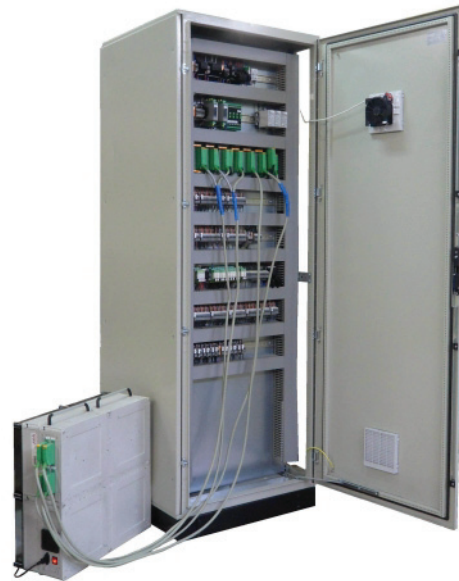
Figure 3 - Overview (rear) and method of connecting turbine control cabinet (right) with hardware simulator (left)
