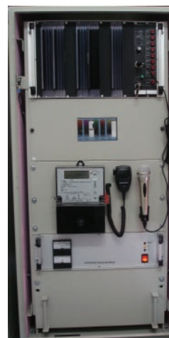
Alarm station – Inner schedule of equipment
